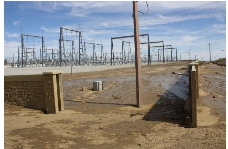
Windhub Substation - Tehachapi District
